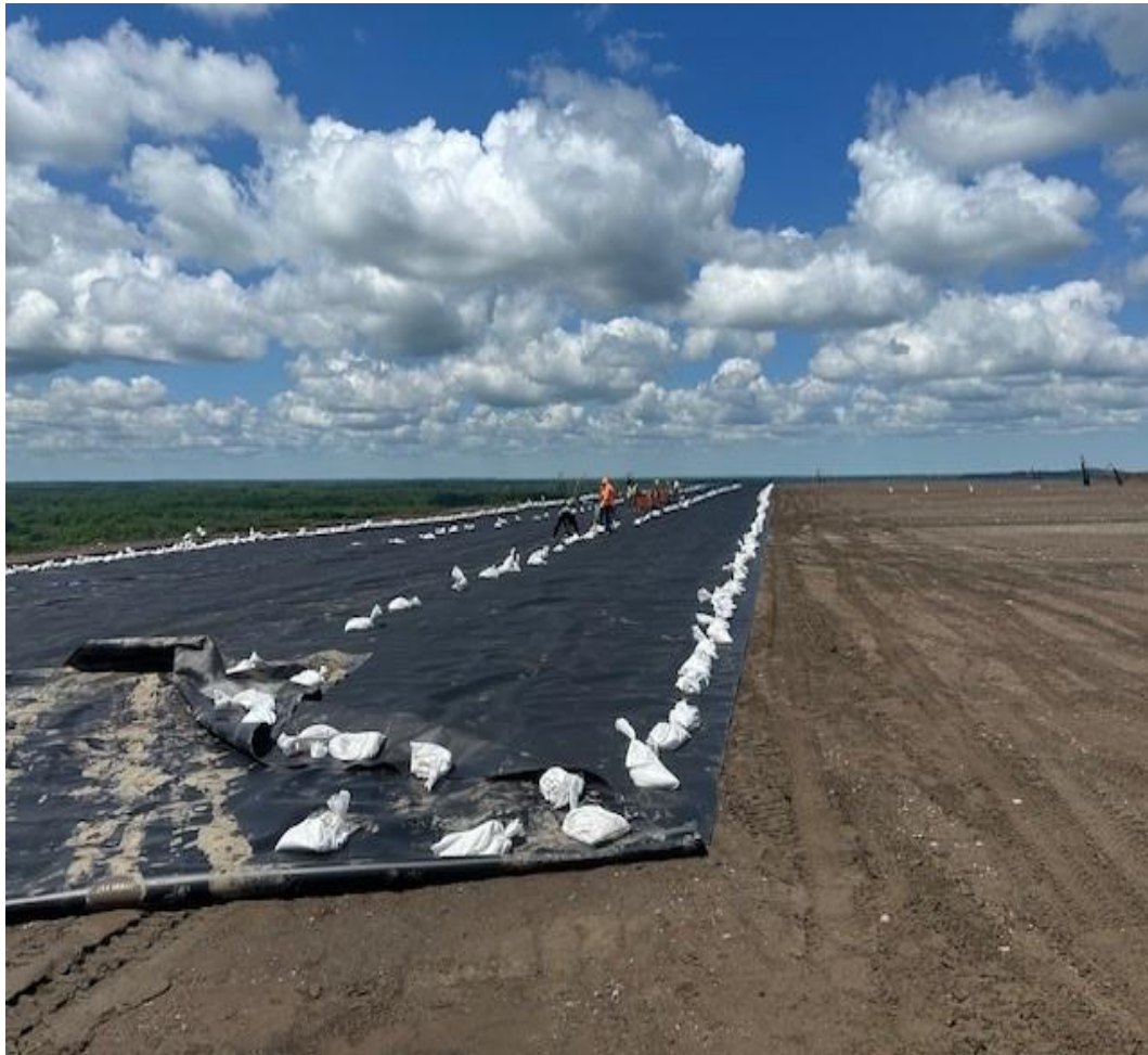
40-mil Geosynthetic Material
