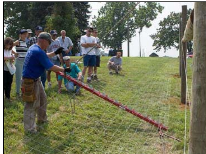
High-tensile woven wire deer exclusion fence installation workshop conducted at NJAES Cream Ridge Research & Extension Center.
