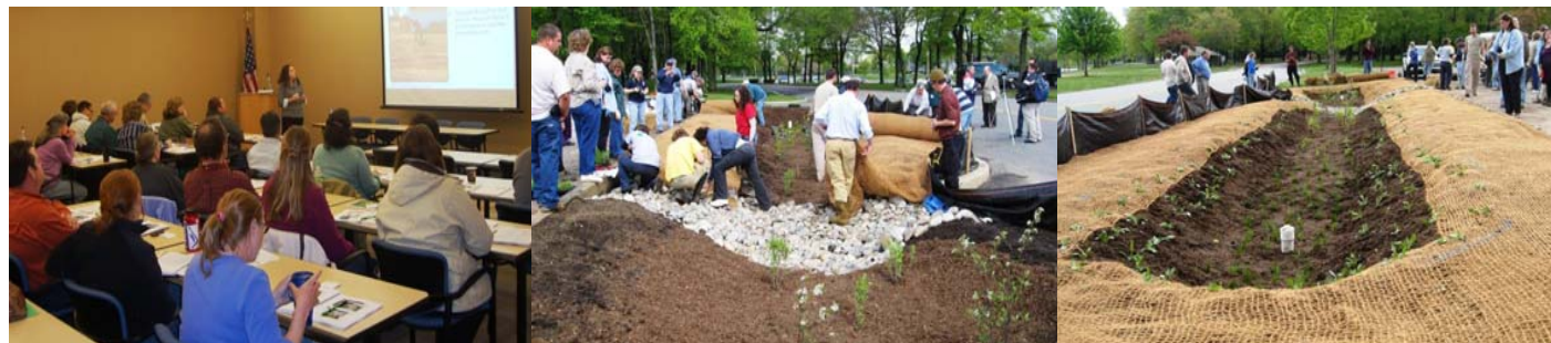
L to R—Michele Bakacs, Cty. Environmental & Resource, instructs in the Ag Building classroom; Next day at Thompson Park, Jamesburg, trainees construct the garden. Stormwater will enter the garden from a curb cut, flow over the rocks which will slow the velocity and filter sediment/pollutants before going into the ponding area. Weed mat will help prevent soil erosion as grass grows in.
