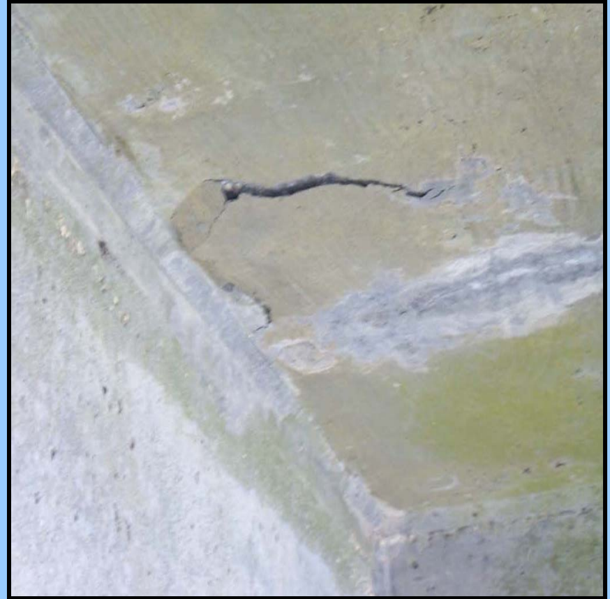
Underside of Deck, Span 4, Under North Sidewalk, Looking Southwest. - Priority I Repair: Large Incipient Spall.
