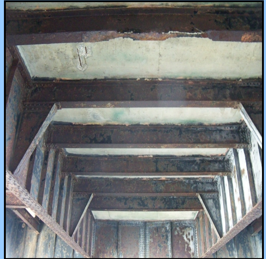
Eastern flanking span (Span 7) superstructure, heavy corrosion and rusting of floor beams, section loss of one floor beam
