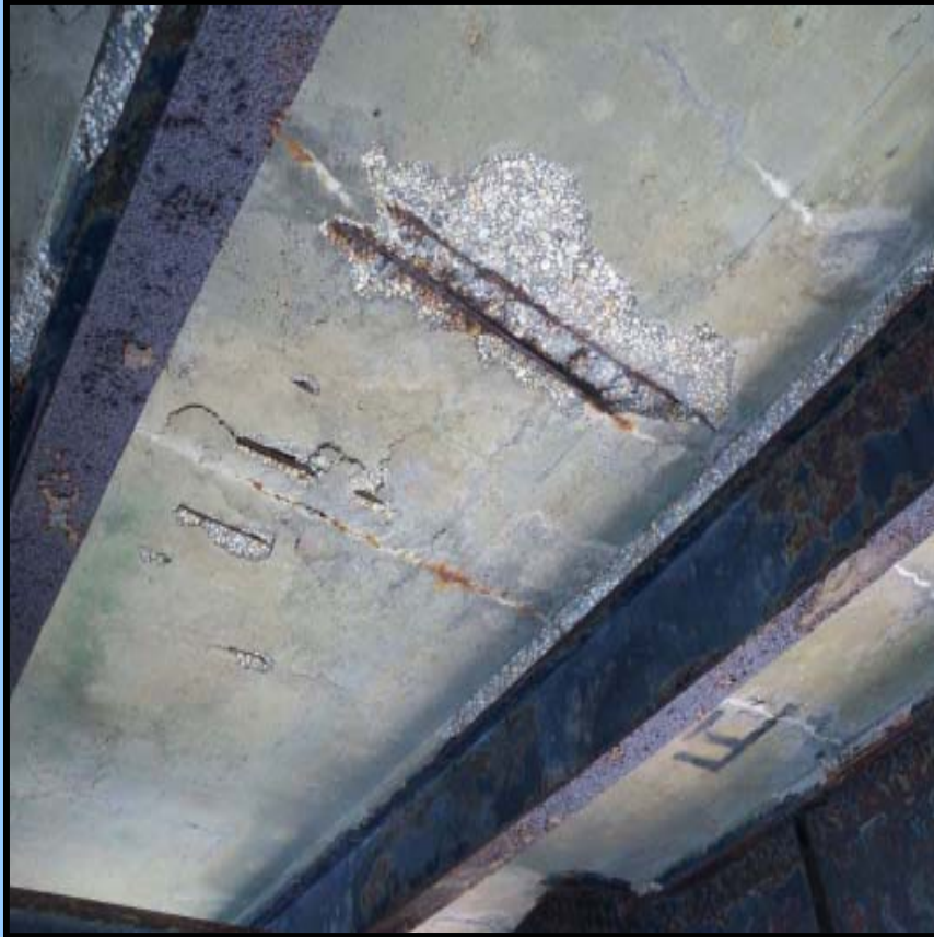
Underside of Deck, Span 4, Bay S2, West End, Looking Southeast. - Large Spall and Incipient Spalls With Rusted Corroded Rebars. Insert: Large Incipient Spall in Bay 2, East End.
