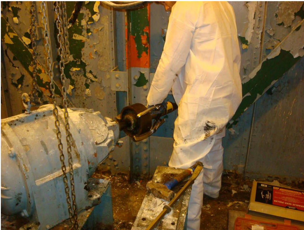
Photo 28: North leaf machinery components; machinery and motor brakes, couplings and brake hubs have been removed.
