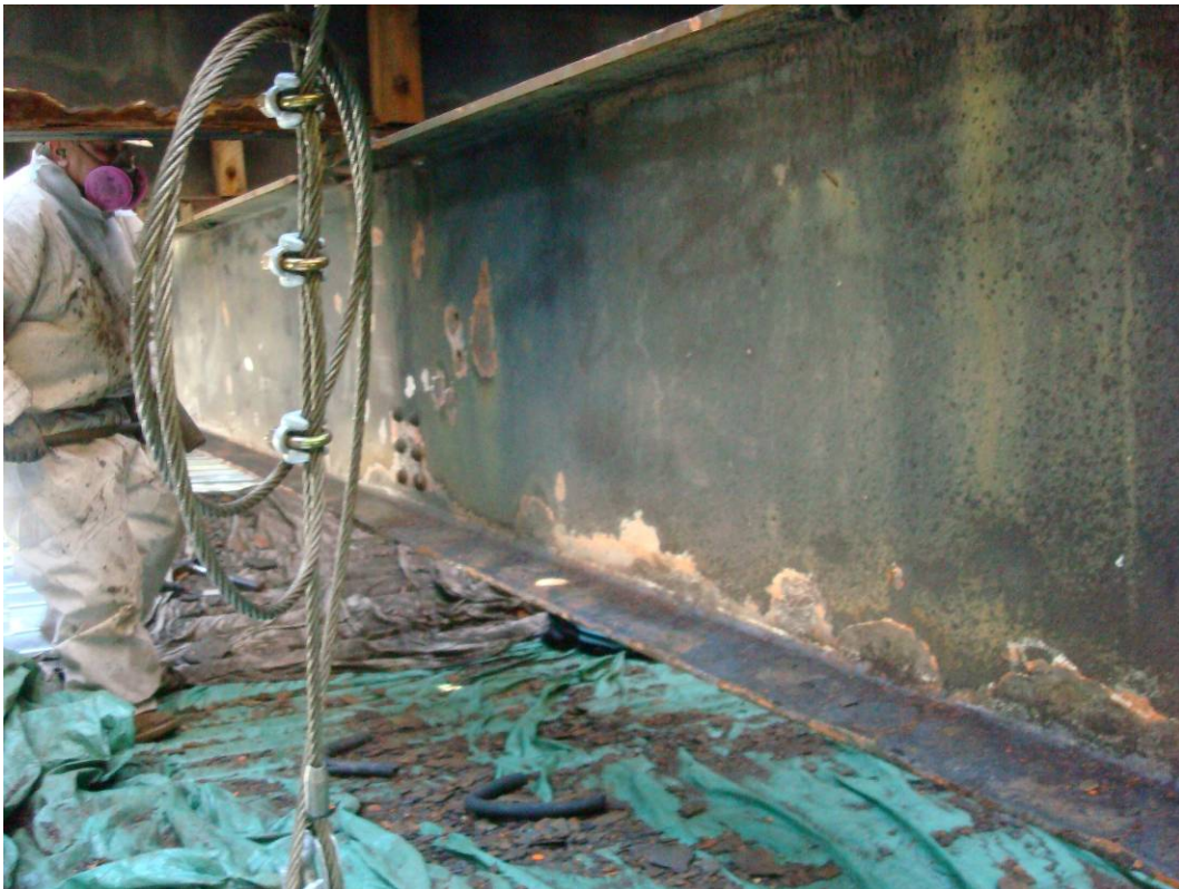
Photo 13: North face of Intermediate Floorbeam FB2 cleaned with hand and power tools.
