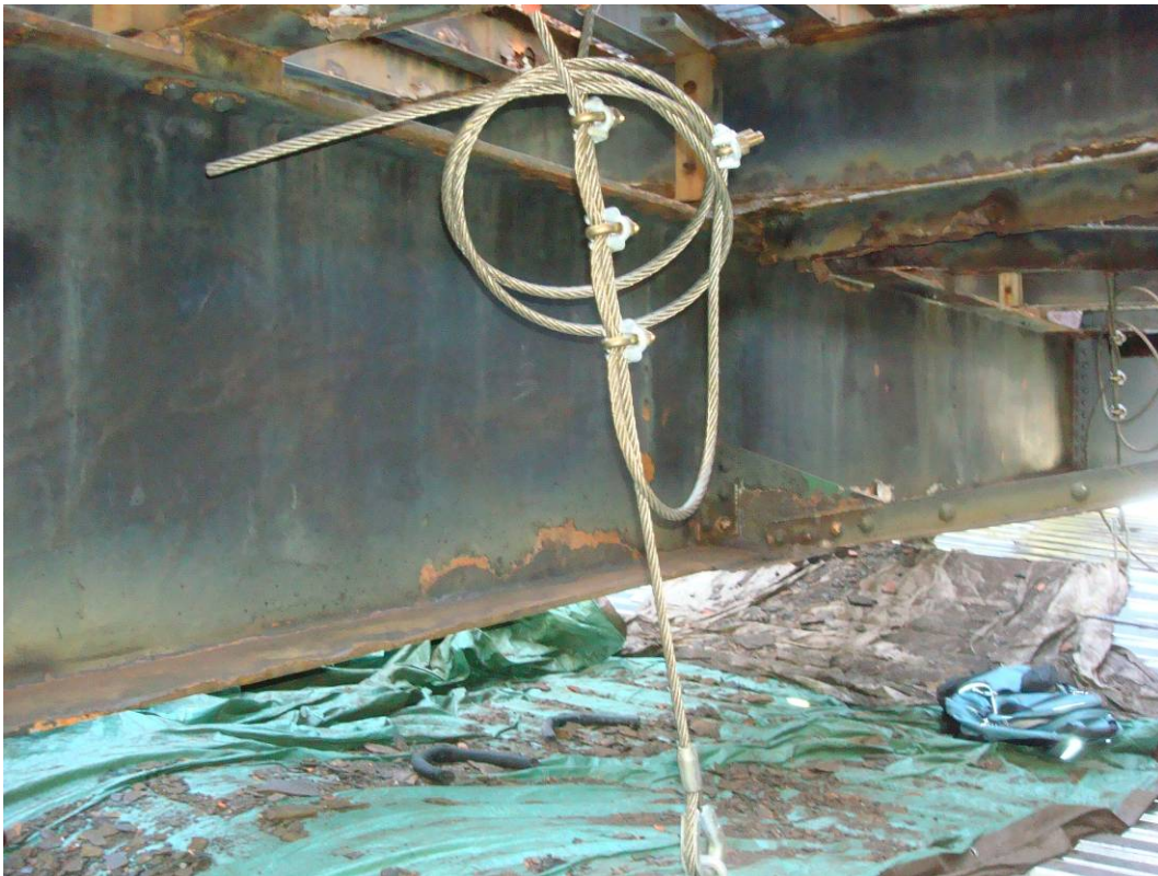
Photo 14: South face of Intermediate Floorbeam FB2 cleaned with hand and power tools.
