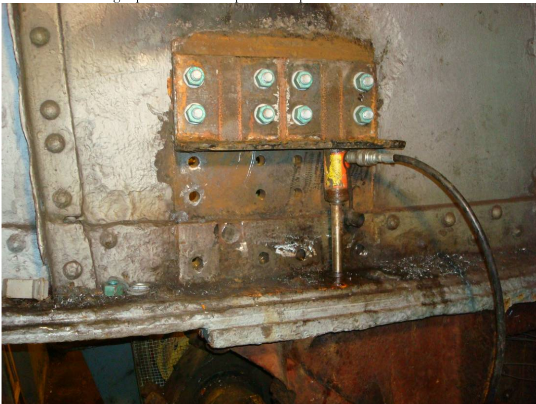
Photo 25: West Bascule girder at the span side rack stiffeners. Stiffeners have been removed and a temporary angle with a hydraulic press is being used to remove the remaining portion of the rack bolts from the bottom flange.
