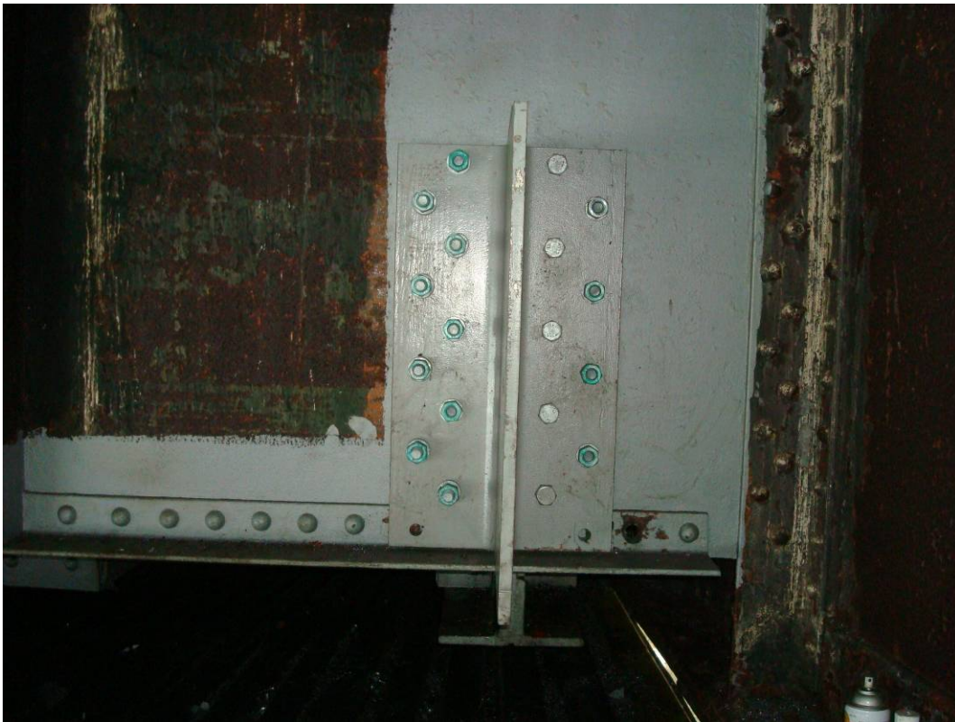
Photo 24: West Bascule girder and Floorbeam FB5, Temporary tie down in position and bolted to FB5 and the Bascule girder. East bascule girder similar. H.S. Bolts between FB5 and Bracket to be replaced with the correct length prior to bascule span FB4 replacement.
