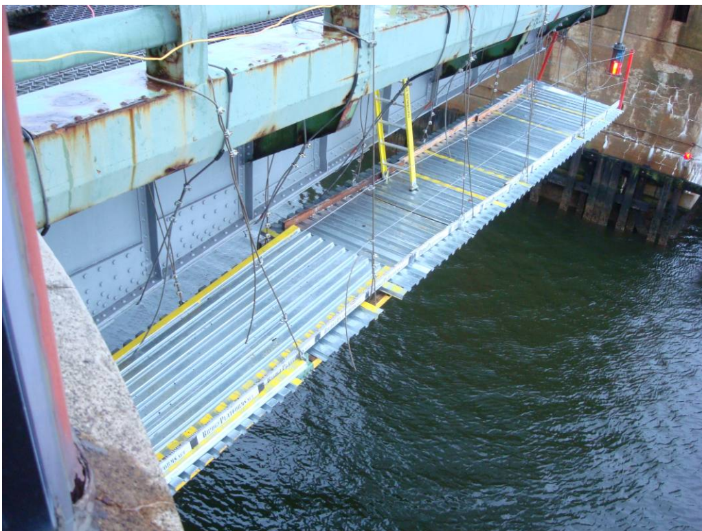
Photo 7: Temporary platform at West side of Bascule span under the cantilevered brackets. Note the bascule girder has been cleaned and primed.
