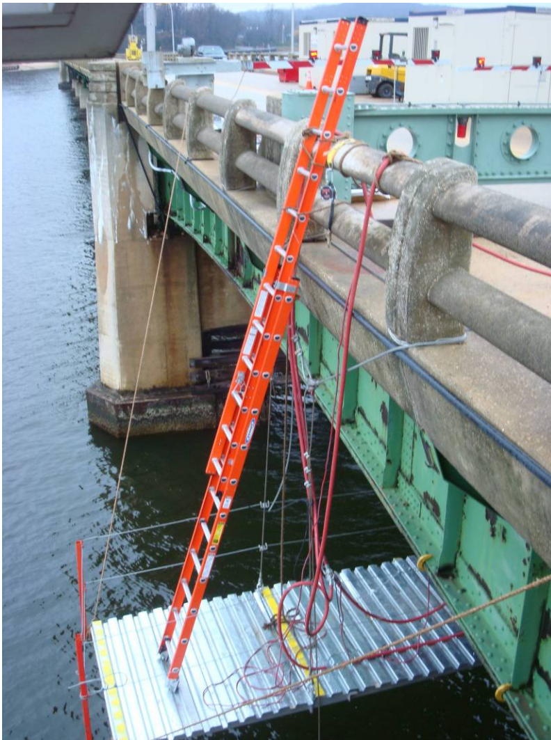
Photo 9: Temporary platform at West side of North Flanking span. Access required for Floorbeam FB5 strengthening and installation of temporary bascule span tie downs.
