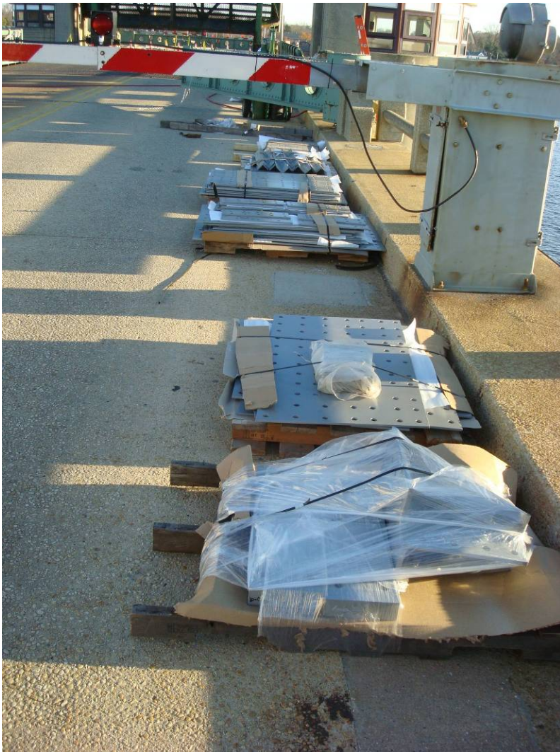
Photo 27: 2 nd Steel Delivery- 6 pallets consisting of 90% of the bascule girder repair plates for both the north and south leafs.
