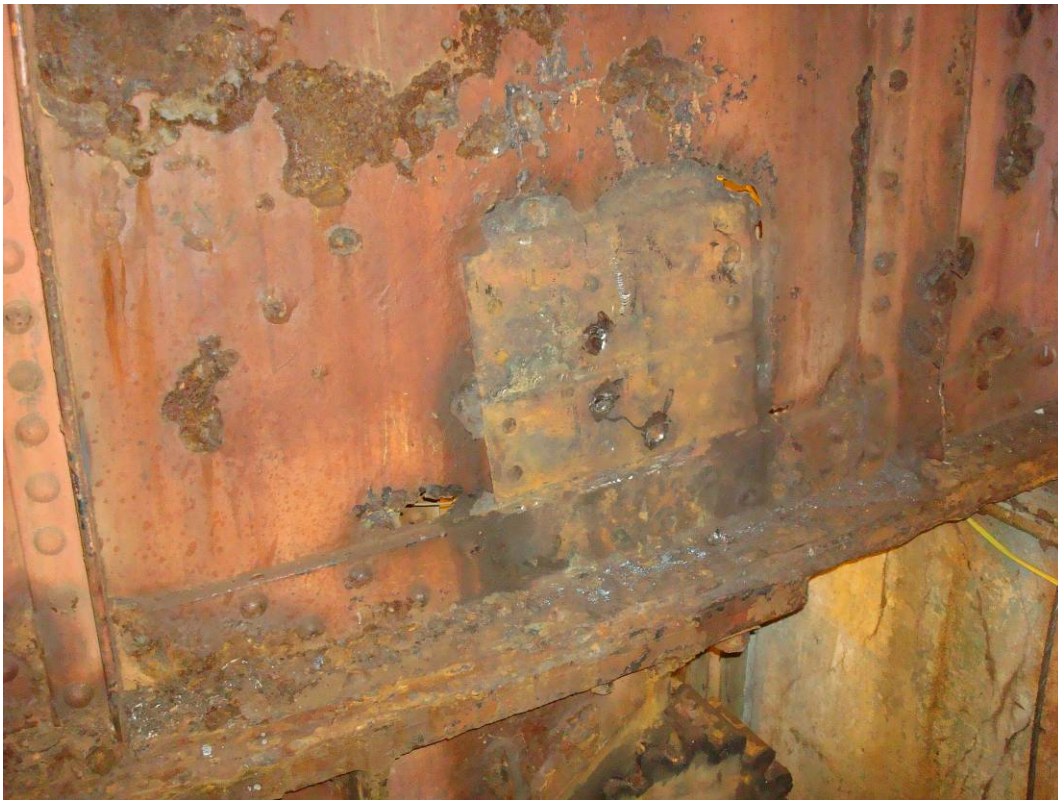
Photo 26: East Bascule girder at the span side rack stiffeners. Stiffeners have been removed from one face only since three rivets remain to be removed as well as the remaining portion of the rack bolts within the bottom flange. Iron workers moved to the west girder while this section of the bascule girder will be hand and power tool cleaned and primed by the Painters.
