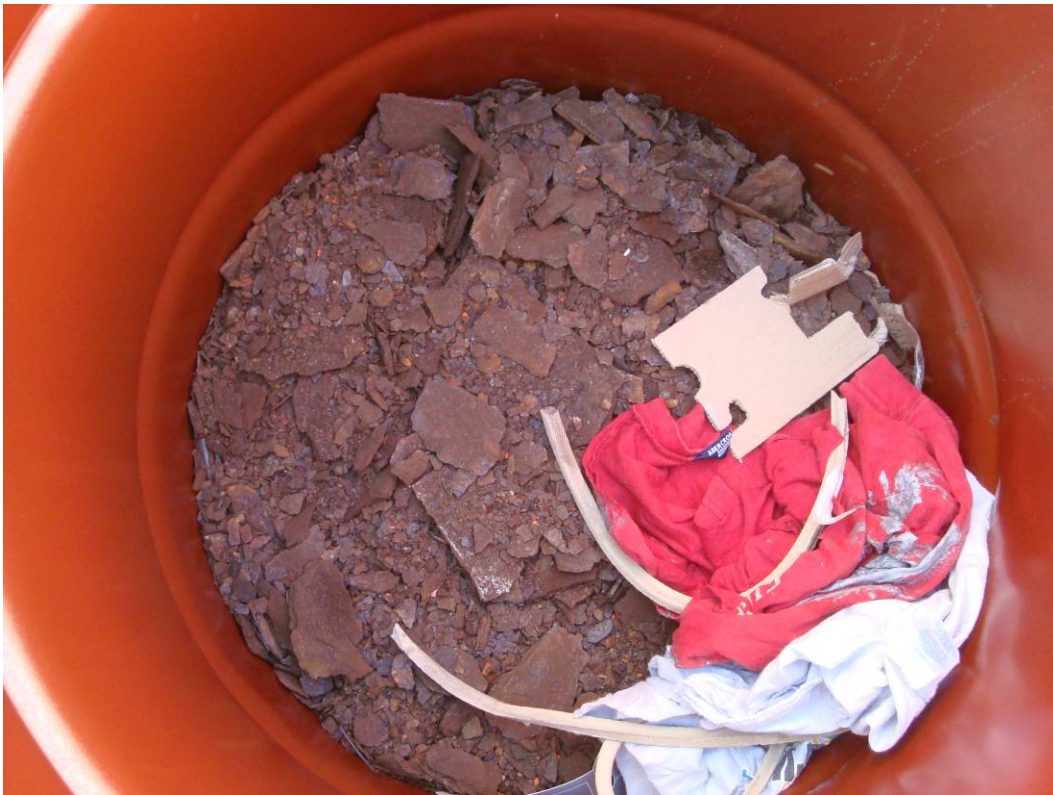
Photo 10: Collection of debris from the hand and power tool cleaning, approximately 7500# of rust has been removed to date on the north leaf and flanking span.
