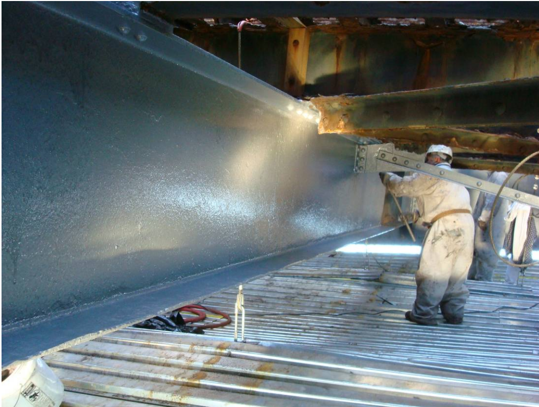
Photo 16: South Face of Intermediate Floorbeam FB3 primed with Epoxy Mastic Aluminum. Stringers and lateral bracing not painted to be replaced.
