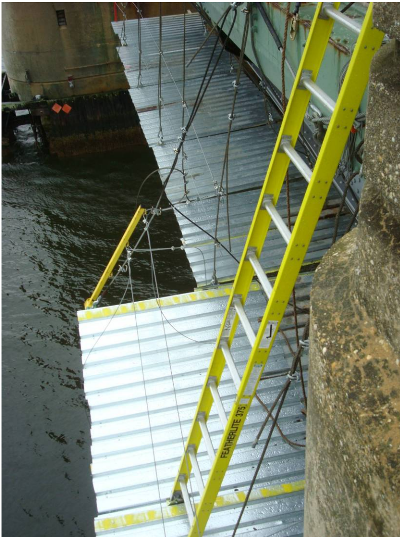
Photo 8: Temporary platform at East side of Bascule span under the cantilevered brackets. Note the bascule girder has been cleaned and primed.
