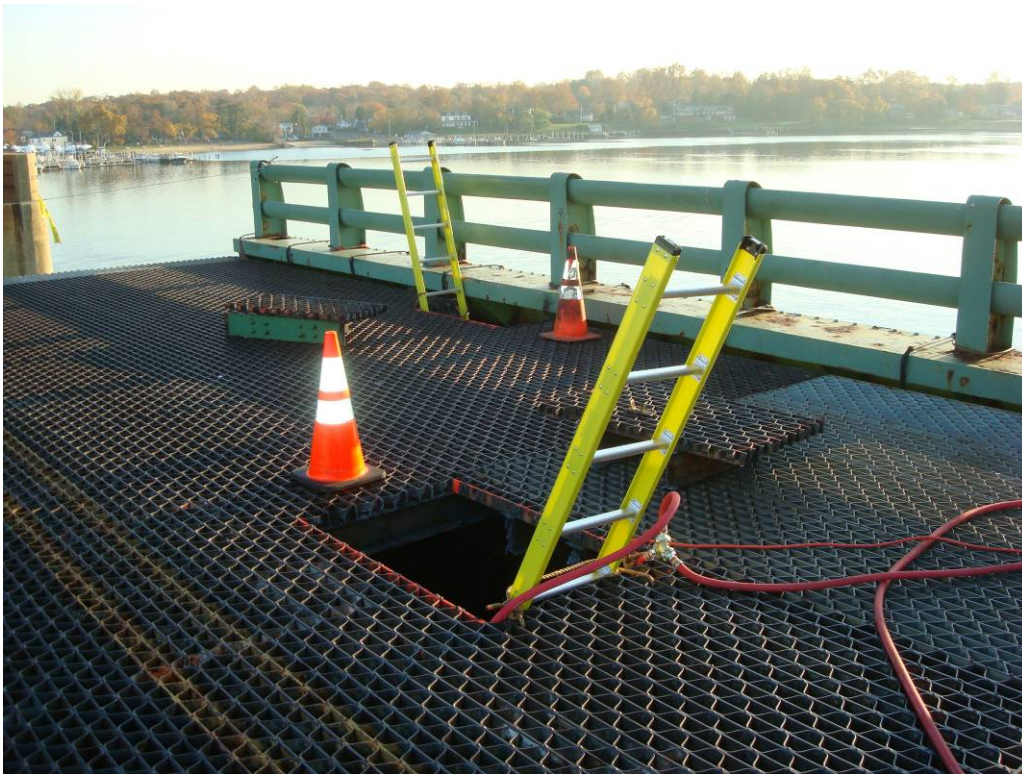
Photo 6: Access openings in North leaf grating deck. Background opening accesses the west cantilevered brackets. Foreground opening accesses between the girders.
