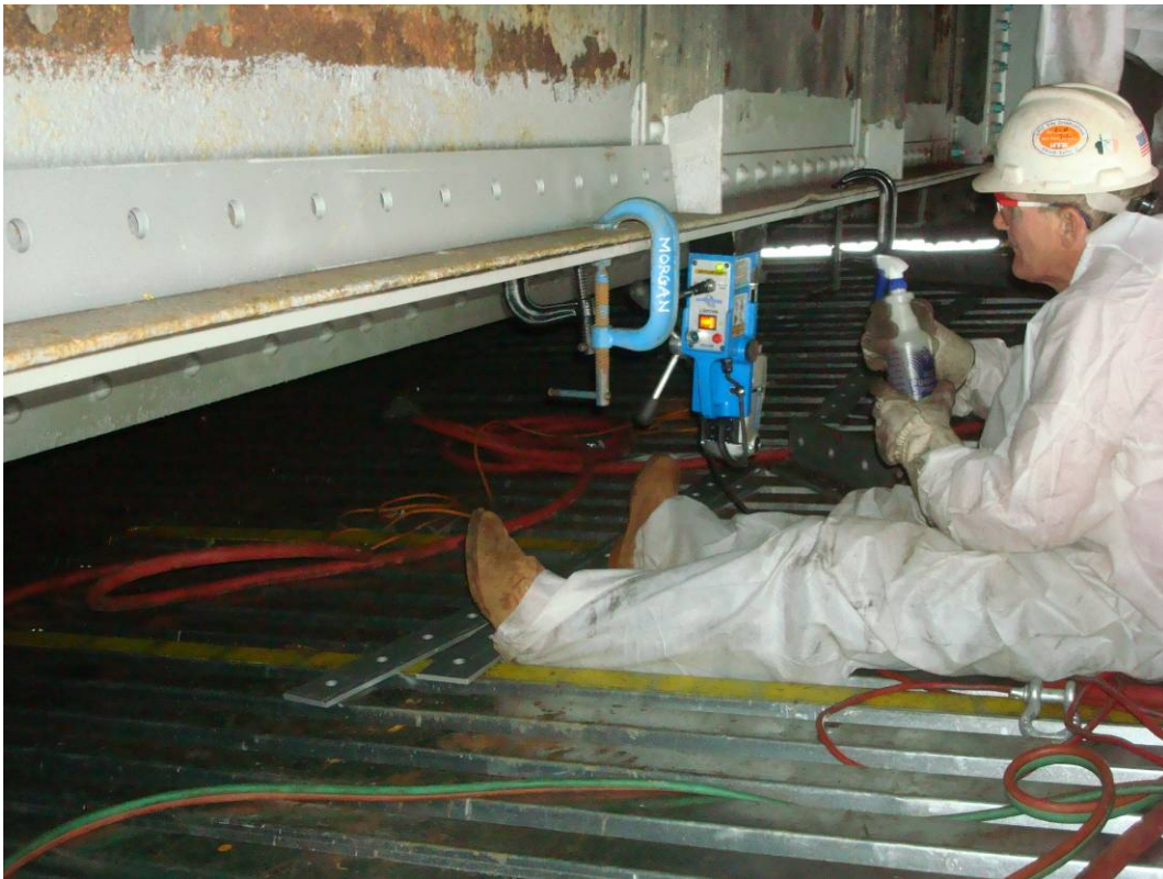
Photo 20: Floorbeam FB5, Field drilling of existing steel using the new cover plates as a template.
