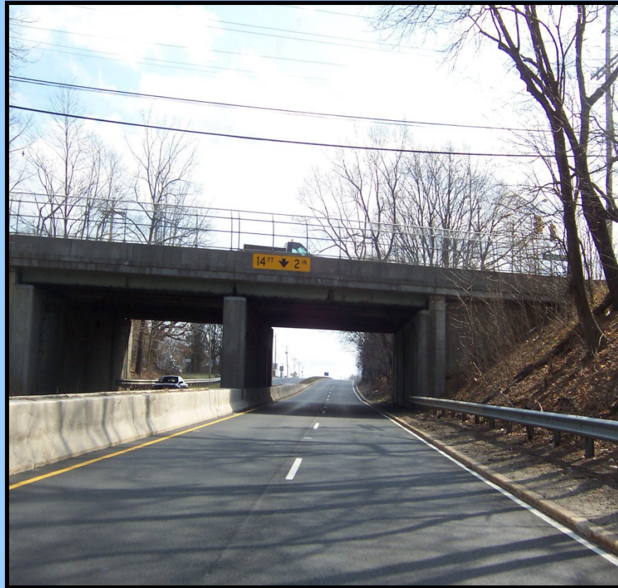
Substandard Vertical Under – clearance at Route 537 Bridge over Route 9
