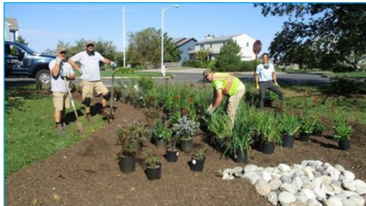
Monmouth Beach Department of Public Works staff and Sara Mellor, Rutgers, installing a rain garden this fall.
