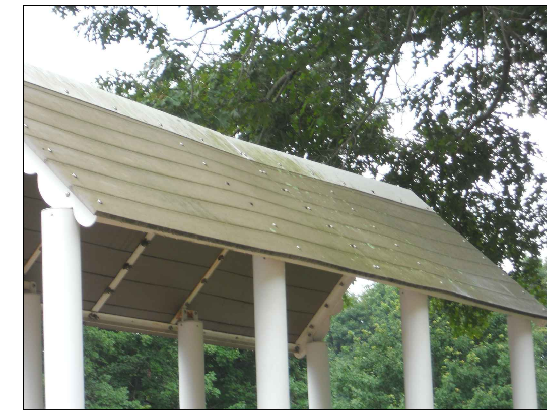
Mold on top of shelter roof.
