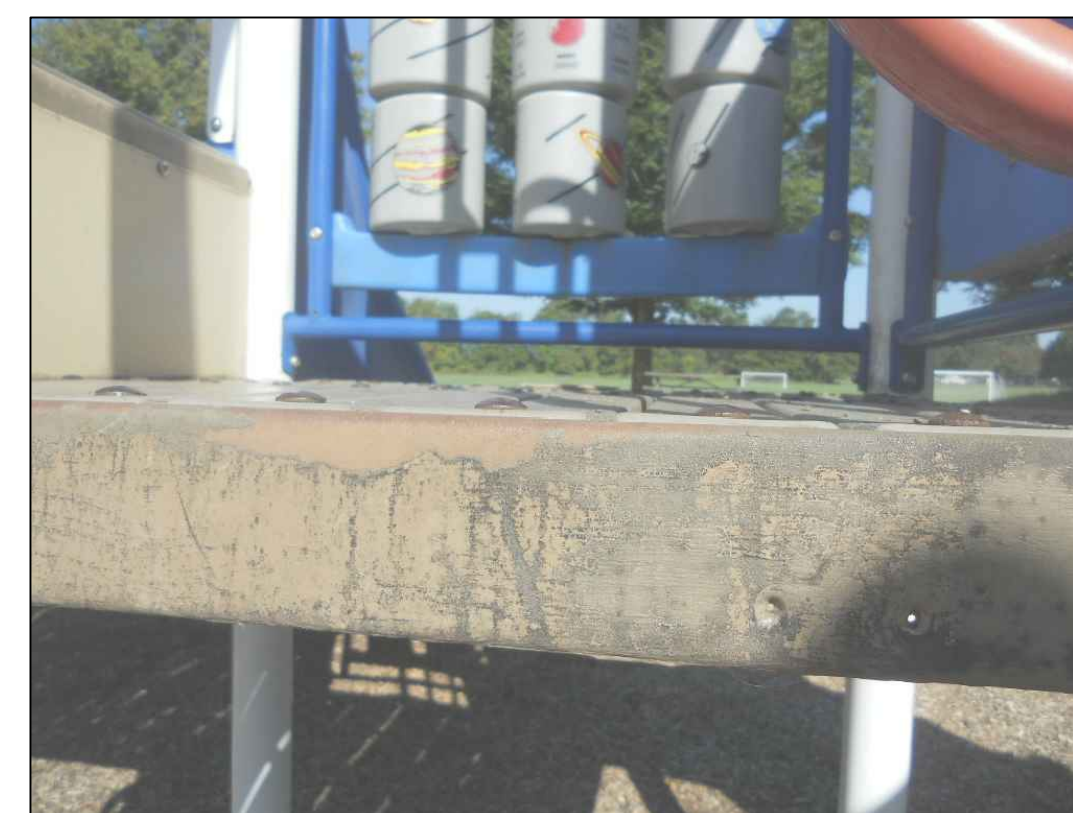
Mold on platform edges.
