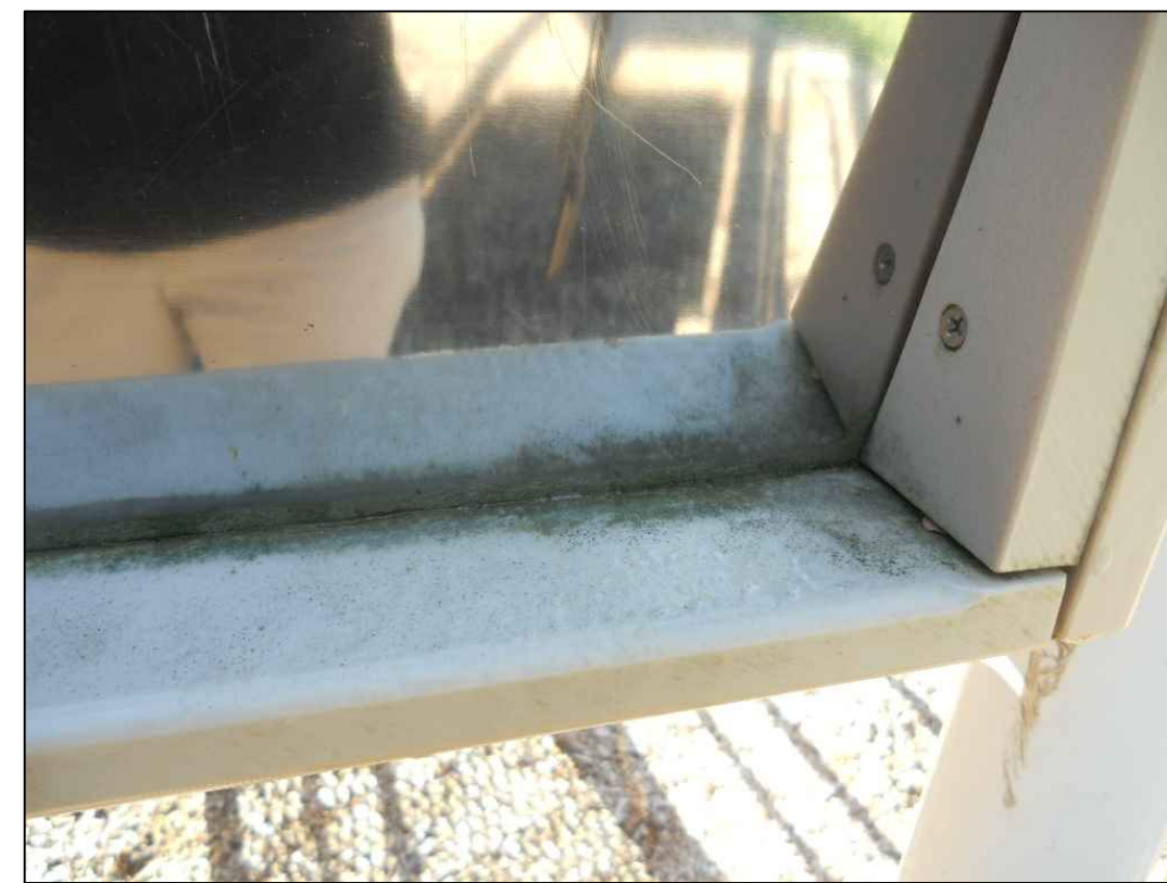
Mold and dirt on posts on panel frames.
