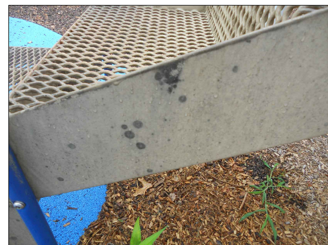
Mold on sides of stairs.
