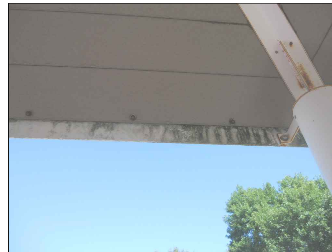
Mold on underside of shelter roof edge.
