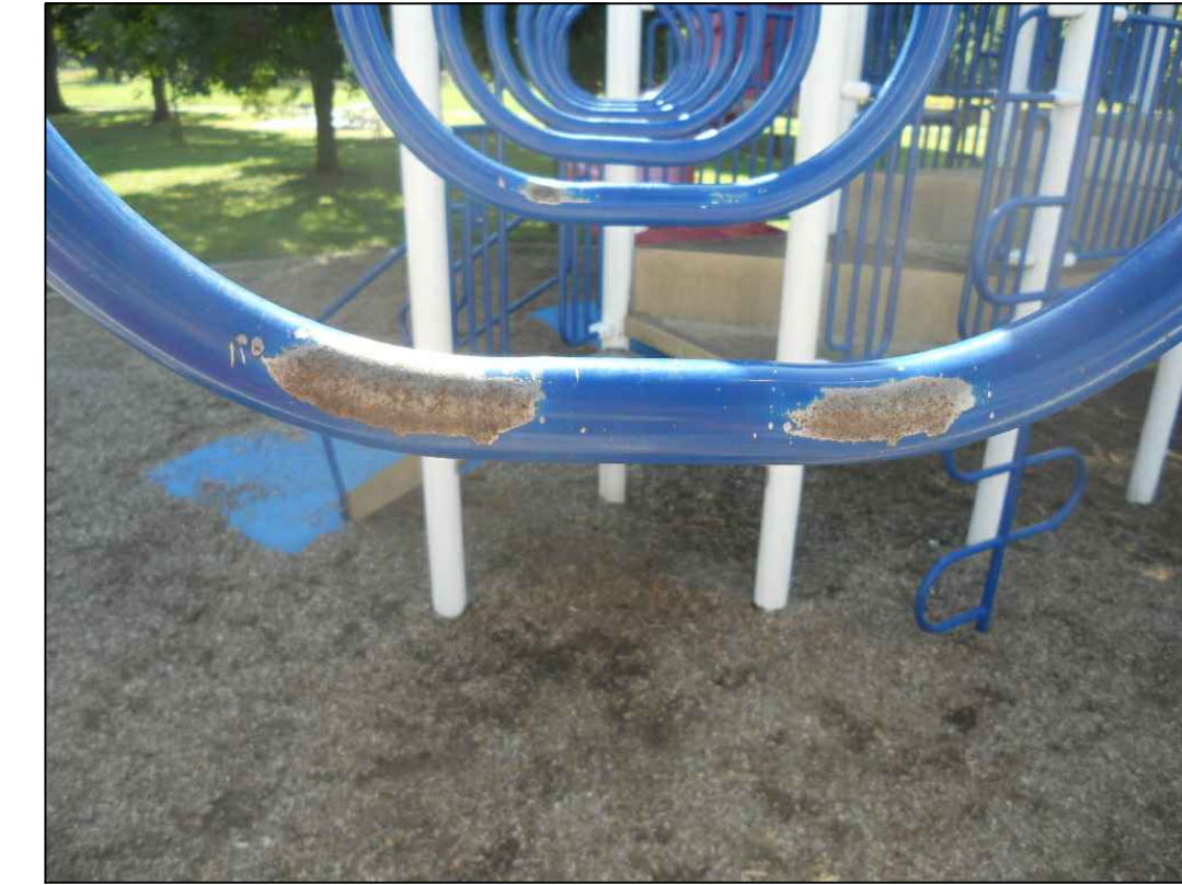
Repair areas on the metal play equipment where rusted or worn; sand, prepare and apply primer and paint with color matched GameTime® paint.
