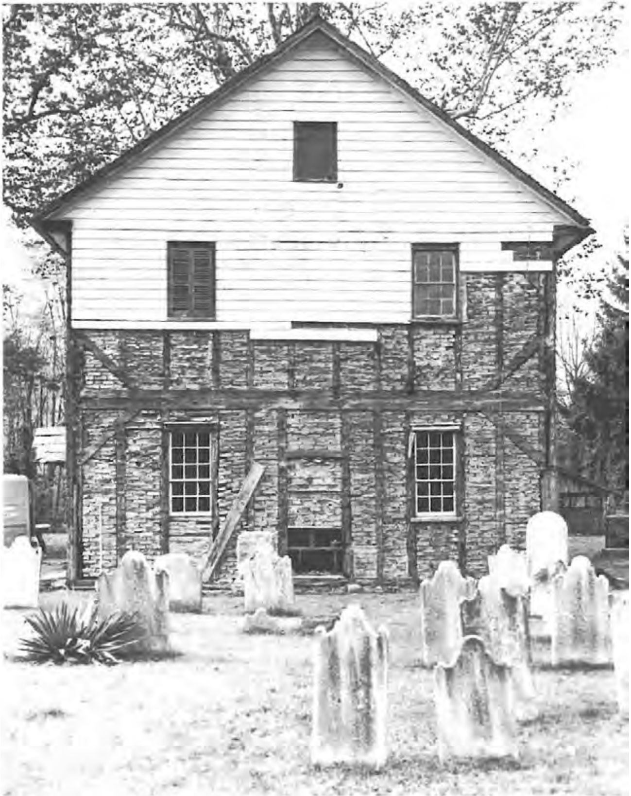
Upper Freehold Baptist Meeting (MCHSI 1351-79), in process of restoration. Photo courtesy Monmouth County Historical Association
