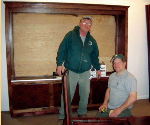
Carpenters Frank Mead and Ray Smith install new cabinets at Tatum Park's Red Hill Activity Center.
