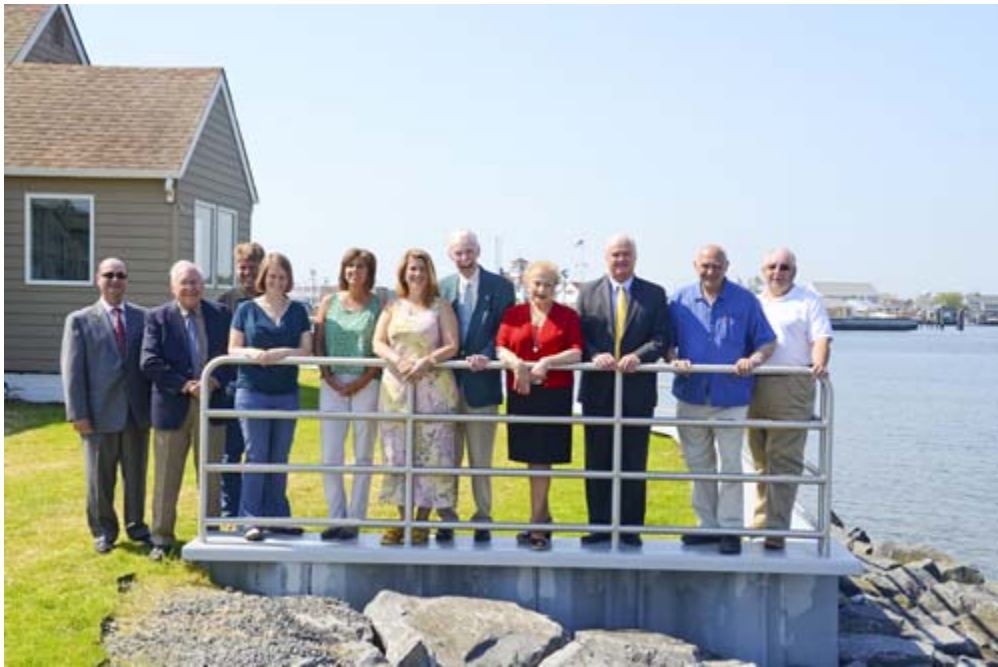
PICTURED – (l to r) Celebrating the completion of the Fisherman’s Cove bulkhead are Tom Nicastro, Superintendent of Department of Public Works in Manasquan; Spence Wickham, Monmouth County Park System’s Chief of Acquisition and Design; Jim Hannon of Bird Construction; Jenna Scott, NJDEP Environmental Engineer; Debbie Voelbel, NJDEP Coastal Engineering; Serena DiMaso, Monmouth County Freeholders Deputy Director; Edward J. Loud, Board of Recreation Chairman; Lillian G. Burry, Monmouth County Freeholder; John P. Curley, Monmouth County Freeholder; George Dempsey, mayor of Manasquan; and John Winterstella, former mayor of Manasquan.
