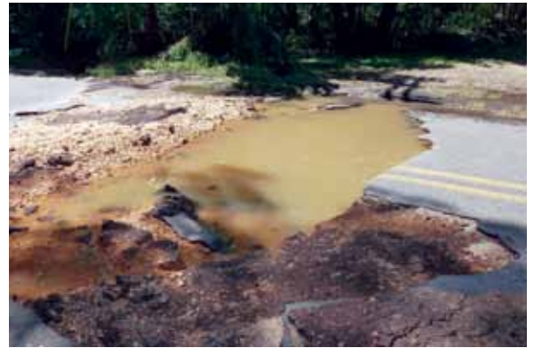
This is what Preventorium Rd looked like after flood-waters receded.
