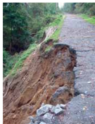
Erosion on the new section of the Union Transportation Trail.
