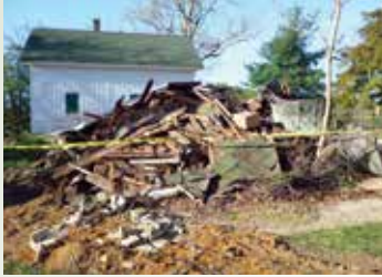
Claypit Creek's leaning silo and shed before and after (that's the Carriage House in the background, currently used for storage).
