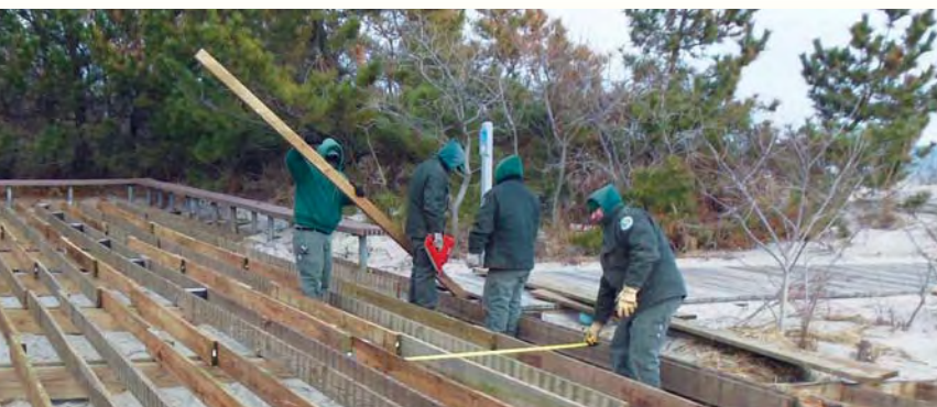
(l to r) Then, Construction & Repair got to work putting the deck together again, rebuilding it from the foundation up. (l to r) Carpenters Dan Desoucey, Ryan Bennett, Chuck Longo & Joe DePierro.
