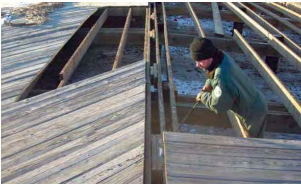
(l to r) Boardwalk repair started with Seven Presidents Park Rangers, such as Pat Becker shown here, pulling up the flood damaged boards, many of which had buckled.
