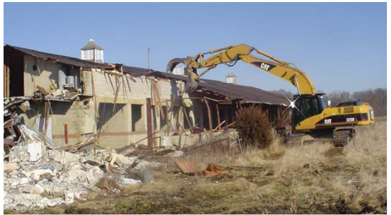
Demolition of an old horse stable on a piece of property acquired for the Crosswicks Creek Greenway in Upper Freehold.
