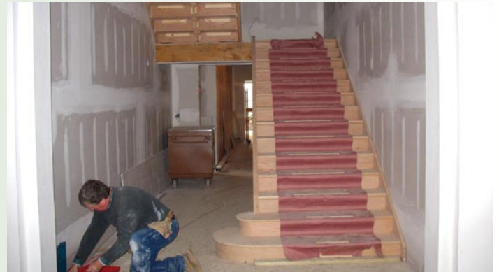
Bought local--Kaufman Stairs of Linden NJ is building the custom "grand staircase" for the new Visitor Center. Here it is, in progress, last November.
