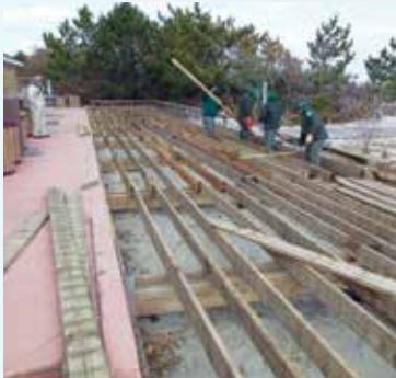
Rangers at Seven Presidents hauled almost 14,000 tons of sand back to the beaches and seawall, in addition to time spent on building and boardwalk repair.
