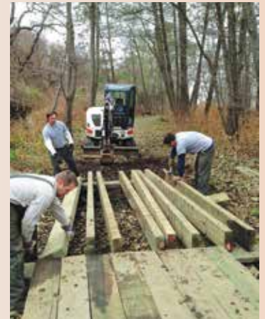
When storm surge from Sandy Hook Bay wiped out all the bridges along the Henry Hudson Trail from Popamora Point to Atlantic Highlands, staff salvaged the wood to rebuild interim boardwalks.
