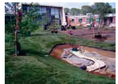
Park staff helped design this water-conserving rain garden in Holmdel, shown here under construction.
