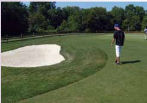
Built by vocational students with some instructional help and support from park staff, this forward bunker made for a lovely “outdoor classroom.”
