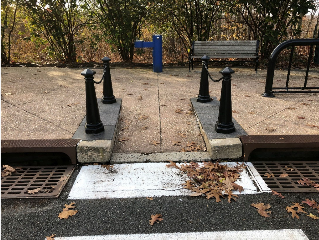
Photo Above: Existing curb and access route to patio to be removed and replaced.
