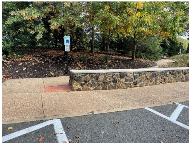
Photo Above: Existing access route to patio to be removed and replaced.
