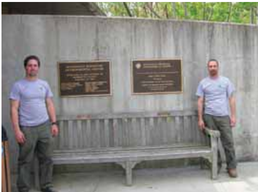
Carpenters Ryan Bennett and Eric Testa install a new plaque at the Manasquan Reservoir Environmental Center to acknowledge grants & gifts from park benefactors.
