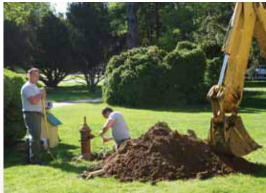
Plumber's Helper Gary Waters (left) and Senior Electrician Mike Vaccaro (right) remove an old fire hydrant from the front lawn of the Visitor Center.
