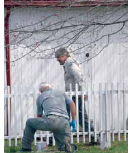
Painters Pat Cernak (kneeling) and Senior Carpenter John Schanck spruce up a picket fence at Longstreet Farm.
