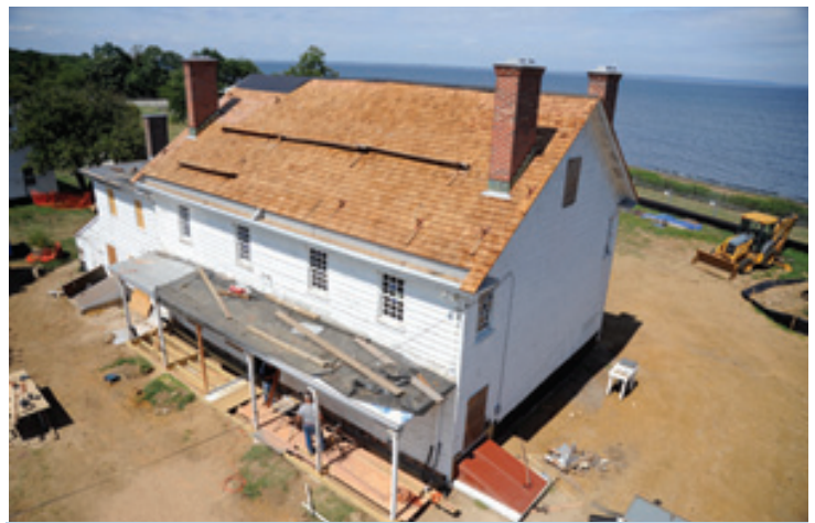
This photo, taken from a nearby crane during the reconstruction, shows the waterfront views of the bay. The New York skyline is visible from this site on a clear day.
