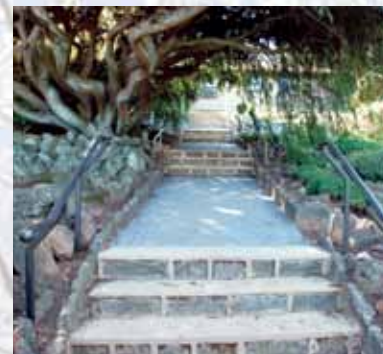
New railings and restored steps make the walkway through the Deep Cut rockery easier to navigate.
