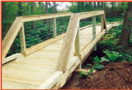
New trail bridges were installed at Shark River Park and Clayton Park (shown).
