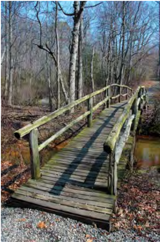
The first trail bridge, built in the early 1960s and likely repaired a few times since then, features carved tree trunks as support beams.
