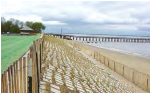
This dune stabilizing 'concrete mat' at Bayshore Waterfront Park proved its worth during Superstorm Sandy.
