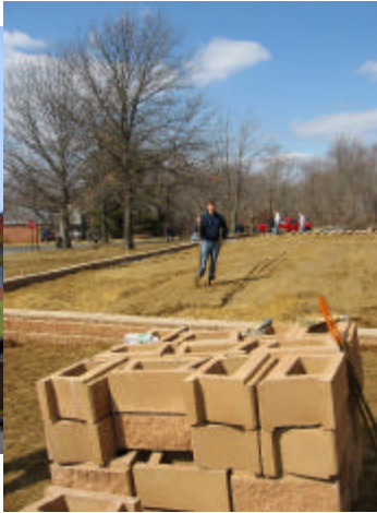
Eagle Scout Jeff Sieminski oversees the construction of a 30' X 90' retaining wall.
